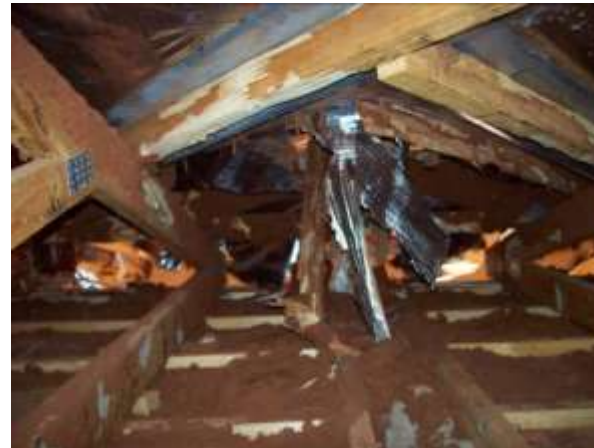
Termites in rafters
