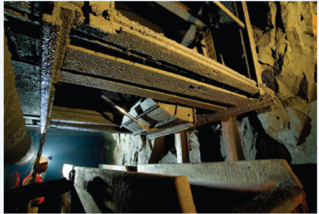
Figure 6:- Details of some engineering solutions being applied to improve safety
